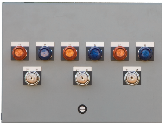
ELECTRIC DERAIL BOX KEYED CONTROL PANEL
